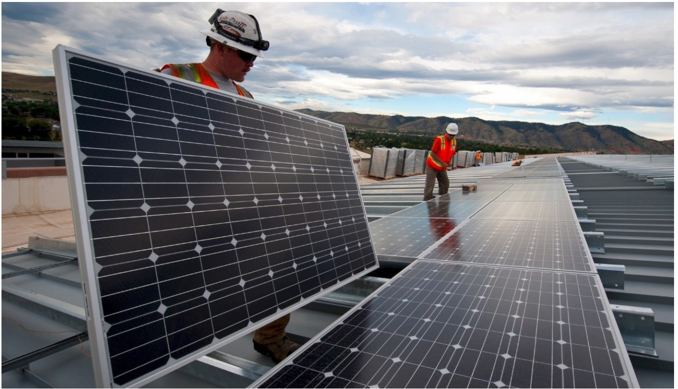
Solar panels being installed on a rooftop. Credit: skeeze via pixabay, CC-BY-1.0
