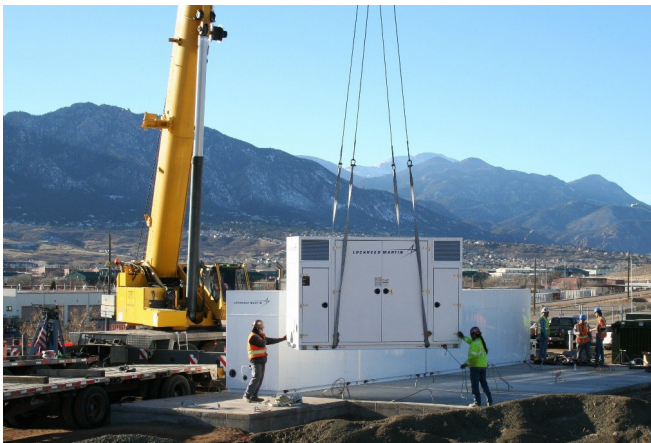
Battery storage being installed at Fort Carson, Colorado. Credit: Scott Clark via U.S. Army Corps of Engineers, CC BY-1.0
